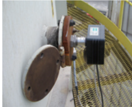
Fugitive emissions on the Furnace Doghouse can also be monitored
